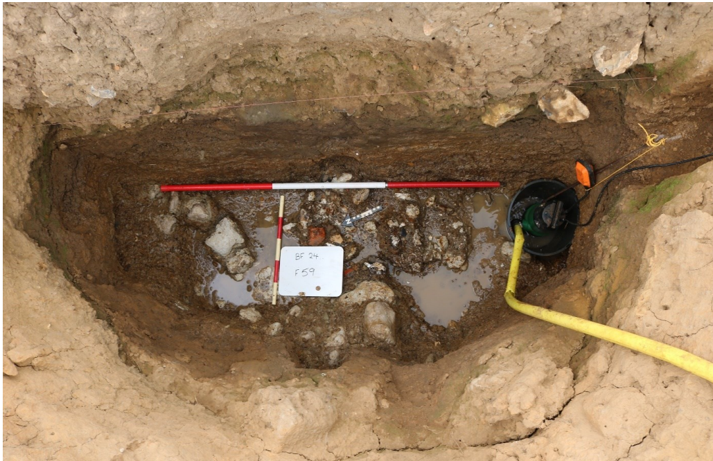
8.79: Chalk and flint revealed due to pumping surface water via an installed sump
